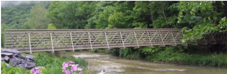
85' x 4' Hiking Trail Footbridge in Loysburg, PA
